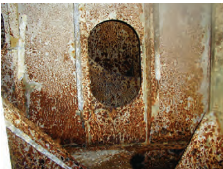
Figure 1: Corrosion in ballast tank on cargo ship.
